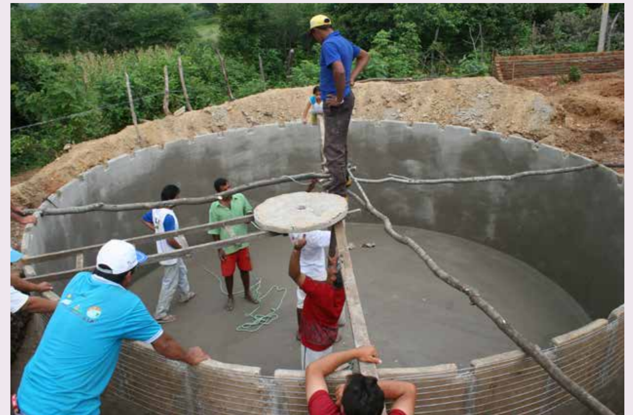
A big scale cistern building-program has given clean water to millions of people in Brazil. These cisterns can contain as much as 52.000 liters of water, and provide farmers with water for their agricultural activities even during long lasting drought. This climate adaptation program has won many prizes due to its successfulness.
